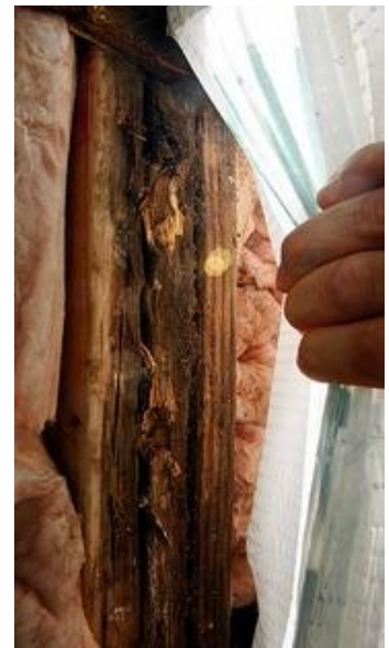
Rotten wood is visible between the exterior and interior walls of the house.
