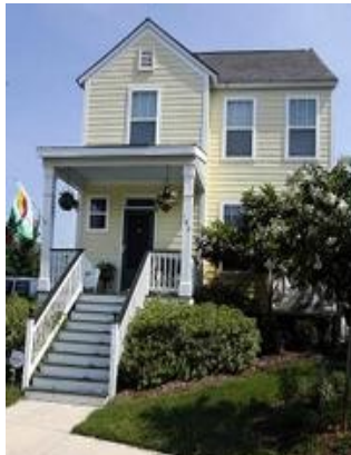
The Allens had their home tested for mold after they noticed it growing on the home's exterior.
