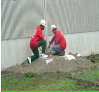
Sand boil at floodwall expansion joint, New Orleans
