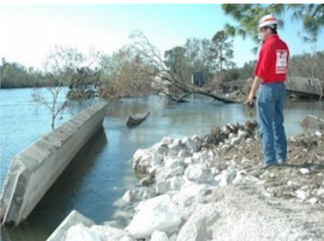
Collapsed floodwall, New Orleans
