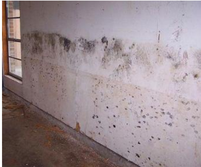
Black mold growing on the wall of a living room in a home that was flooded. (Marie Sanchez)
