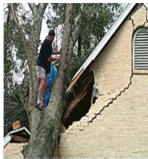
A house in Lake Charles, La., with roof damage after Hurricane Rita.
